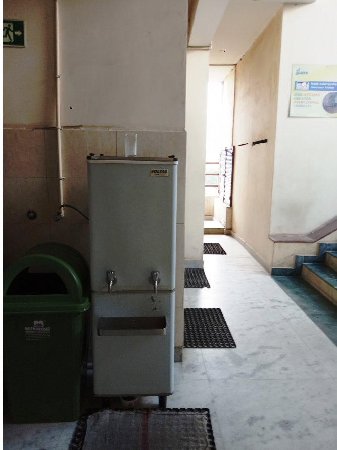
Potable Water, Water Cooler with Ro System
